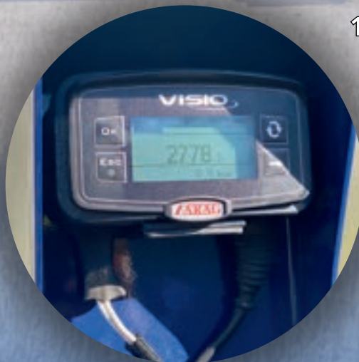
TANK LEVEL SENSOR
